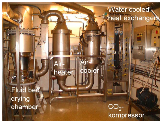
Figure 4 Photo of the laboratory fluid bed dryer with CO 2 as refrigerant
