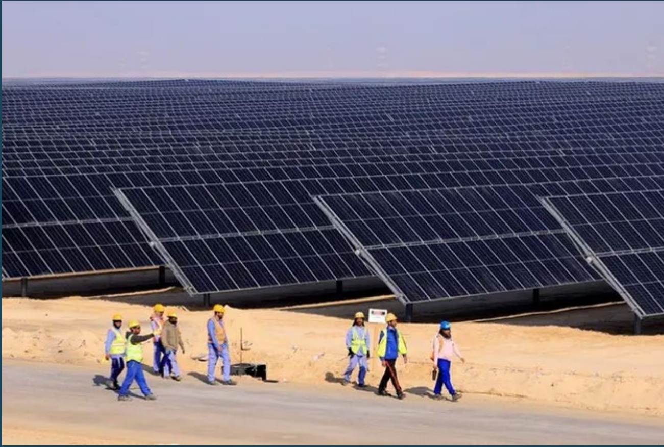
Al Dhafra Solar Photovoltaic (PV) 2GW project, Abu Dhabi (Photo: Karim SAHIB / AFP)
