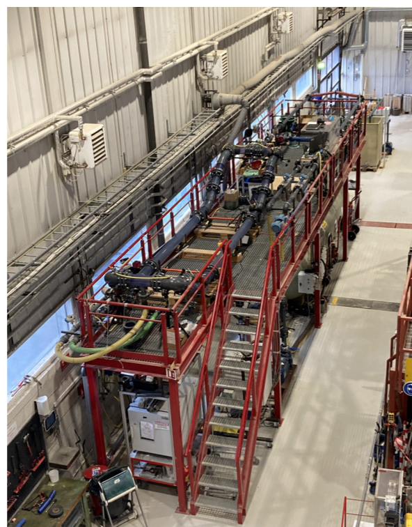
Figure 4a) Photo of the experimental facilities, depicting the separator, control station and flow meters on the top floor and pumps, storage tank on the ground floor.
