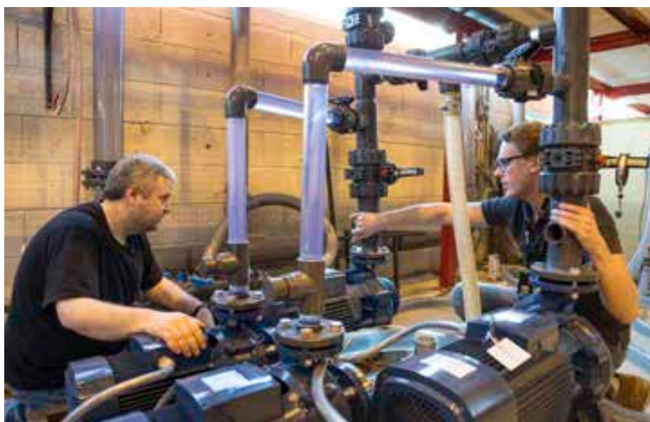
Construction of the compact separator test facility is underway, here with master student Espen O. Hestdahl (left) and PhD candidate Håvard S. Skjefstad (right).
