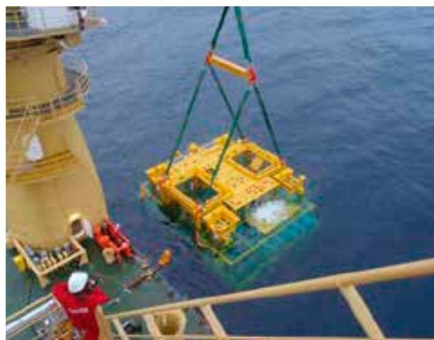
Draugen Subsea Boosting Station – Installation of manifold. Courtesy of AS Norske Shell
