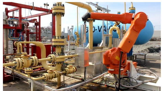
Fig. 9. The valve manipulation operation has been performed successfully tens of times on-site.
