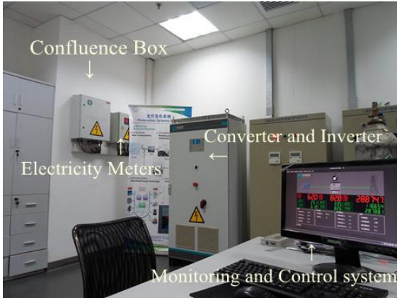
Fig.5 PV system in Department of Automation, SJTU
