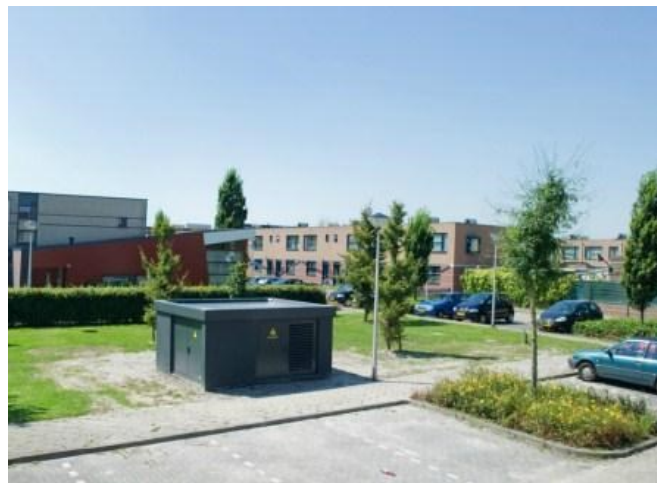
Fig. 1. The Smart Storage unit installed in the field
