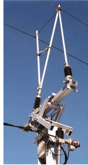
Fig. 2. The mast in the up position with the tilted contact wire
