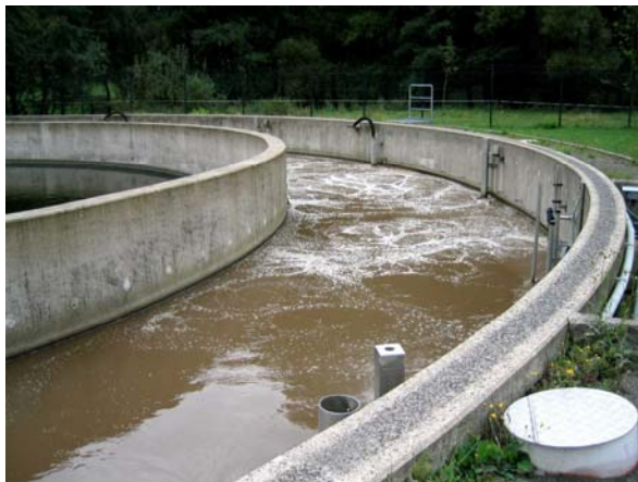
Fig. 1. A intermittently operated waste water treatment plant in Germany
