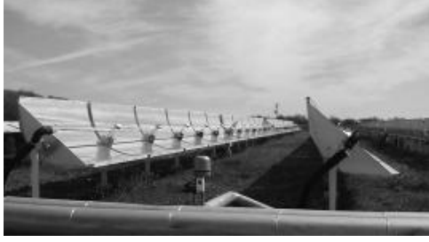
Fig. 1. Solar collectors (one of twenty rows).
