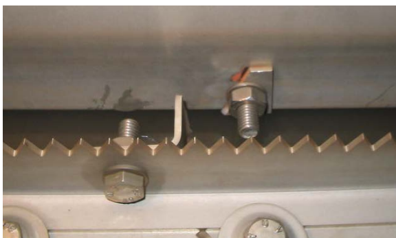
Figure 4: Broken downcomer bracket
