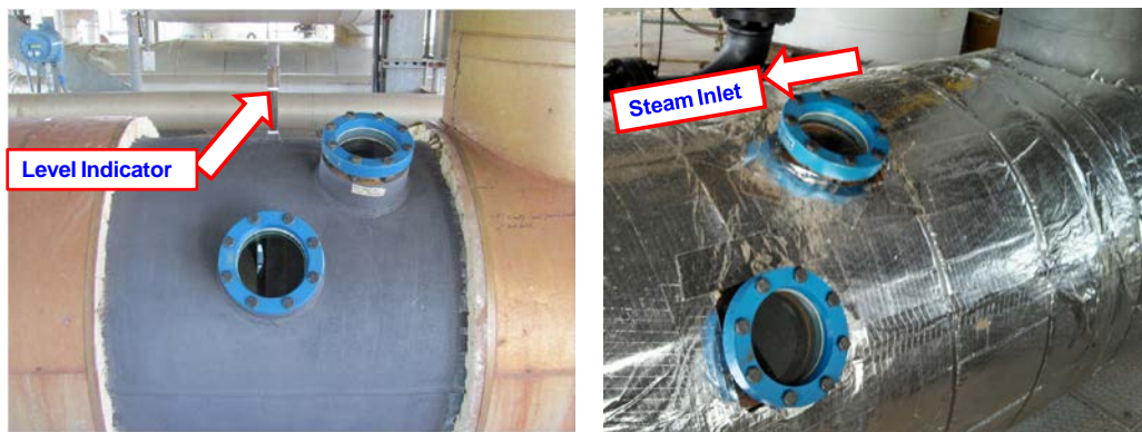
Figure 2. FRI Kettle Reboiler Observation Windows
