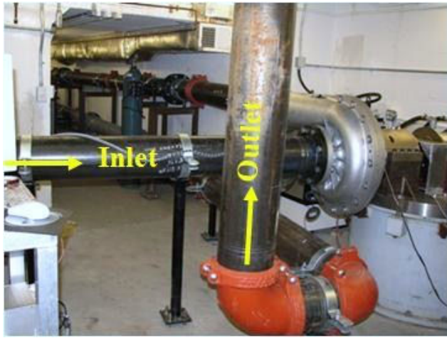
Fig. 1. Photograph of the compressor test rig in inlet and exhaust piping.
