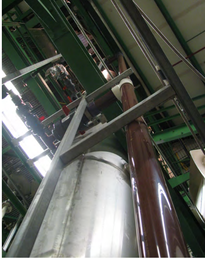
Figure 4: Bubble Column and Transparent External Piping
