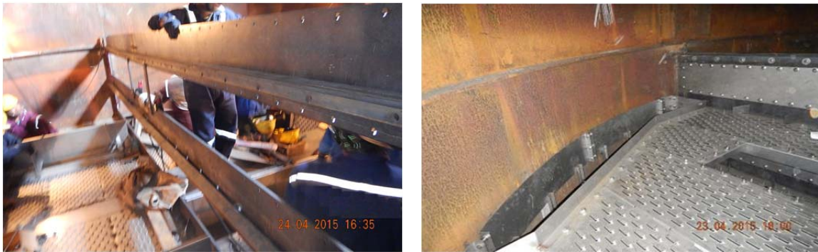
Figure 5a: Installation of the Dividing Wall in the FCC Naphtha Splitter at an Indian Refinery; Figure 5b: Dividing Wall Internals inside the Tower
