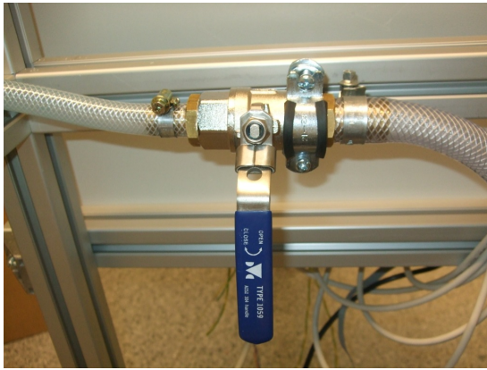
(a) Ball valve at the water inlet.
