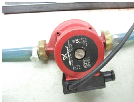
Figure 3.7: Water circulation pump
