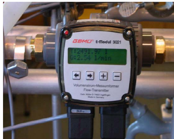
Figure 3.2 Rate meter for water
