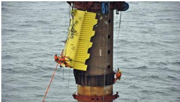
With repair work at full speed during spring, the clamps intended to hold the cables between the platform legs in place, were installed.
