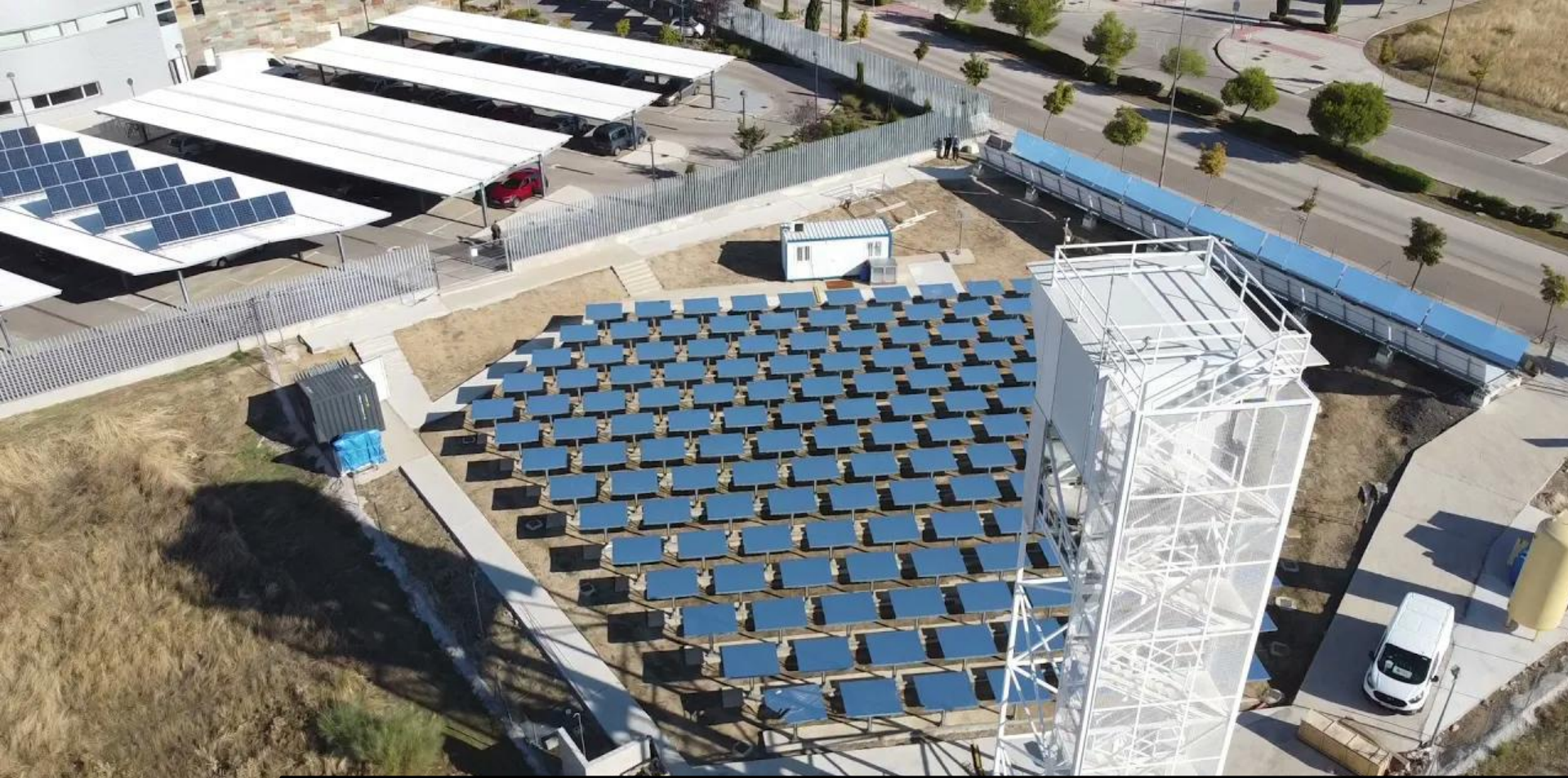
M. Romero, et. al, "Ultra-modular 500m 2 heliostat field for high flux/high temperature solar-driven processes," , 2017
