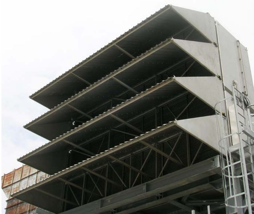
Inlet to filter
