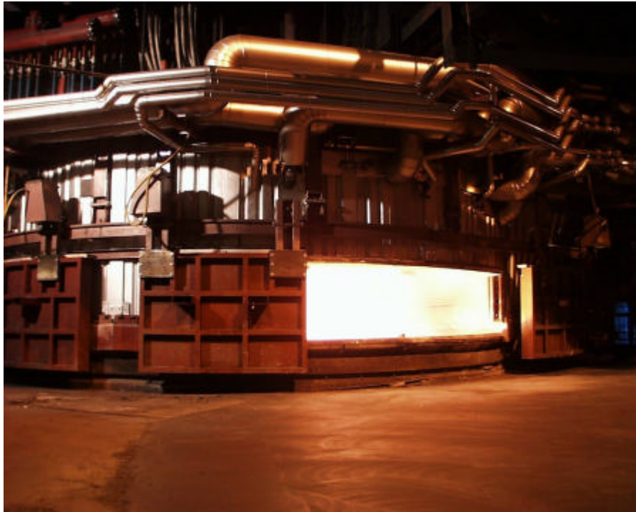
Image 1: Furnace no. 1 at Elkem Thamshavn (Photo: Elkem ASA, Silicon Division)
