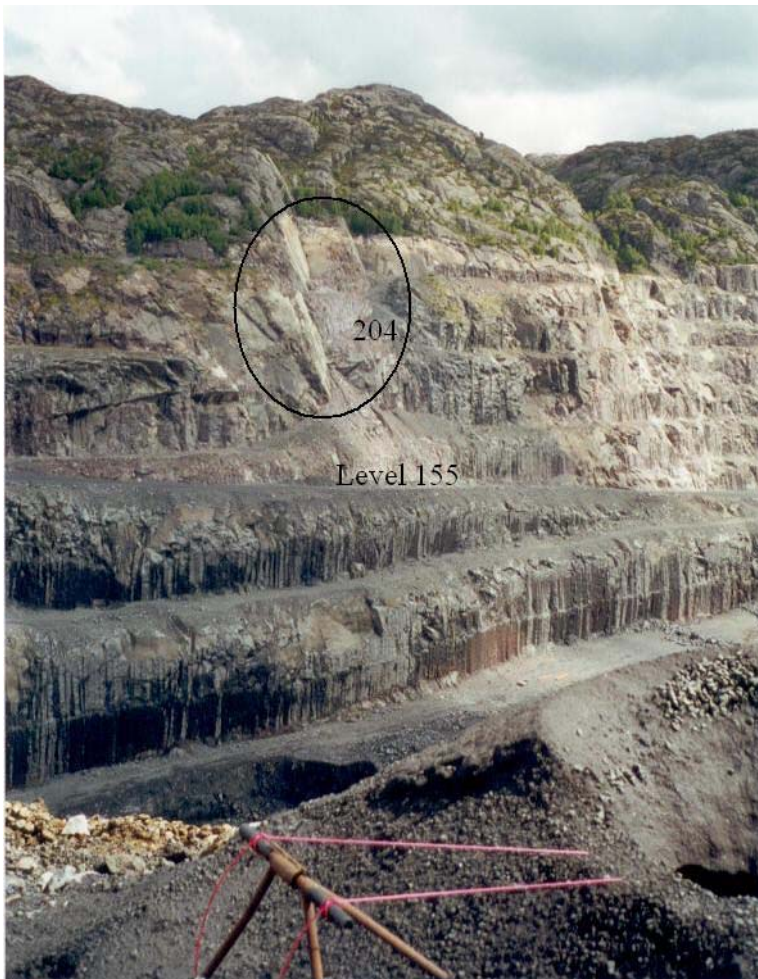
Figure 5. Slide area above the main transport road in the footwall, profile 1150 (photo taken from SW).
